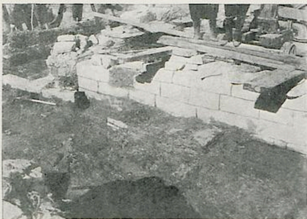
Fig. 16. Foot of the T Foundation abutting on and bonded through the W. wall of A Basis.
